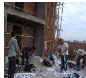
Electricity, security alarm, phone, TV,...
