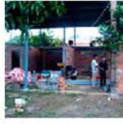
Setting up of a new (2nd) Center in Siemreap-Kantuo. Building site for students and trainers who carry out excavation and construction work.
